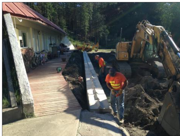
This home next to Texas Creek now has barriers in place to protect against floods.
