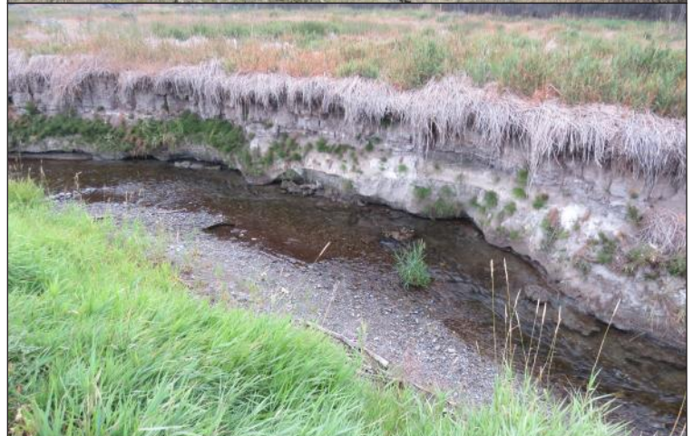
The above photos show the incised channel in the Myers Creek watershed. The streambed has dropped, and as a result, the stream is disconnected from its floodplain.
