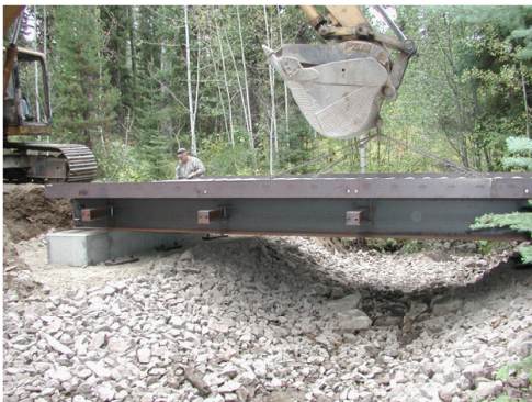
Replaced with a 30' x 12' steel bridge at a cost of $38,000, opening up 3.4 miles of rainbow and bull trout habitat.
